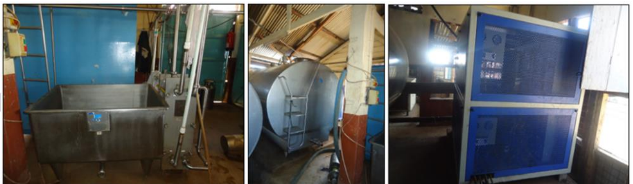
Figure 8. As installed at Olenguruone (see figure above)
