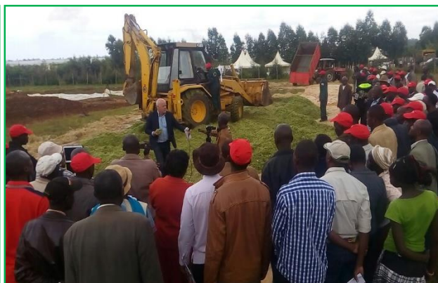
Participants watch as compaction progresses. Weight enhanced tractor was used for this
